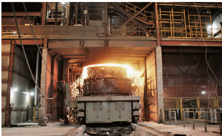
The secondary-metallurgy station at the Kalinganagar plant used analytics to increase throughput by better controlling the superheating process.
